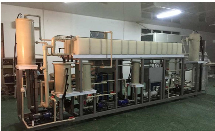
Actual MDS 500 system for FGD wastewater treatment
